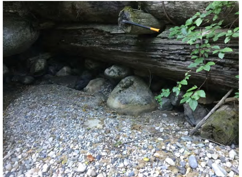
Left abutment downstream scour
